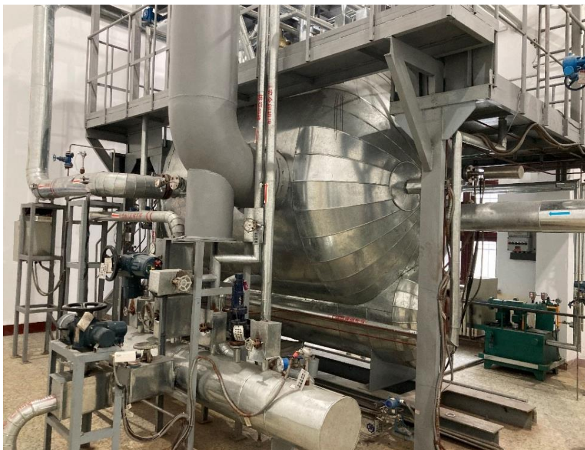
Figure 2. Experimental equipment of experimental supercharged boiler system.
