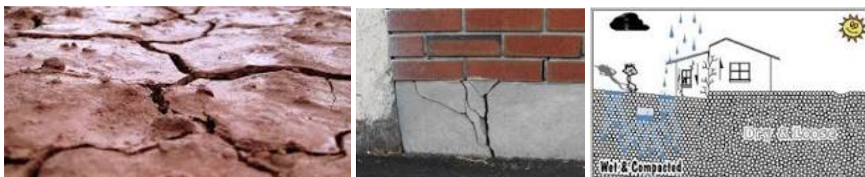
Figure 1. Cracking and uneven foundation.
