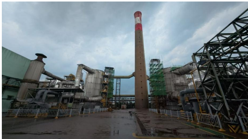
Figure 5. Copper smelter flue gas acid system.
