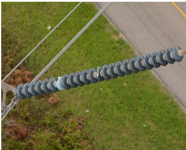
Figure 23. Raw image of defected insulator.
