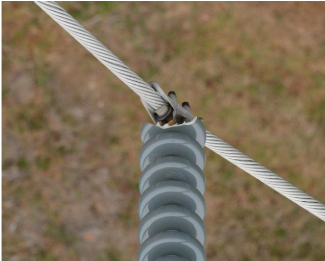
Figure 21. Raw image of broken insulator.
