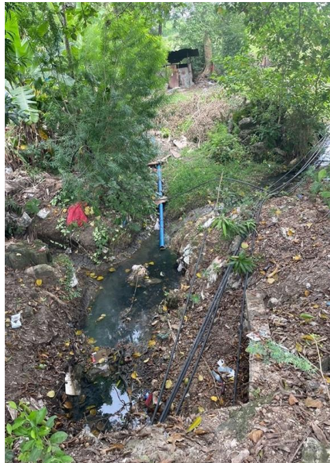
Figure 5. Picture of damaged water pipes, taken by the participants from Chake Chake during the photo elicitation activity.
