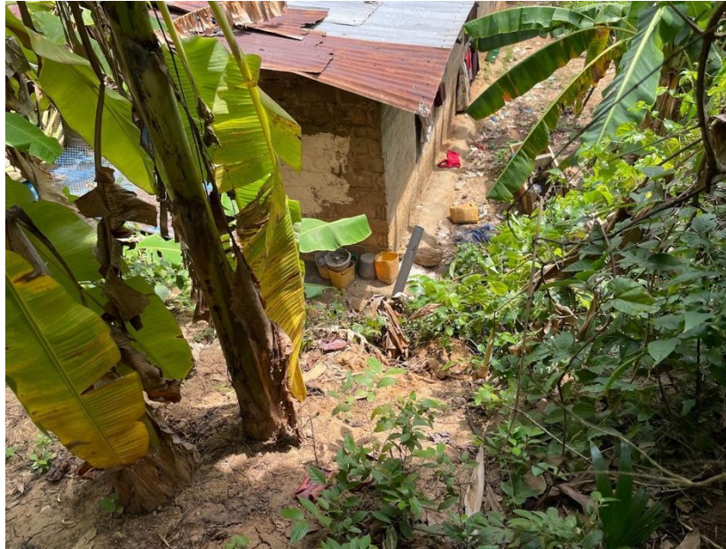
Figure 13. Picture of houses built on unstable terrain prone to landslides, taken by participants from Mkoani during the photo elicitation activity.
