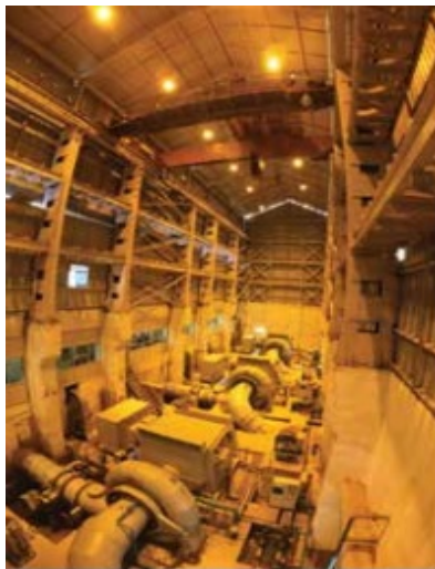
Dikshi 24 MW SHP Power House
