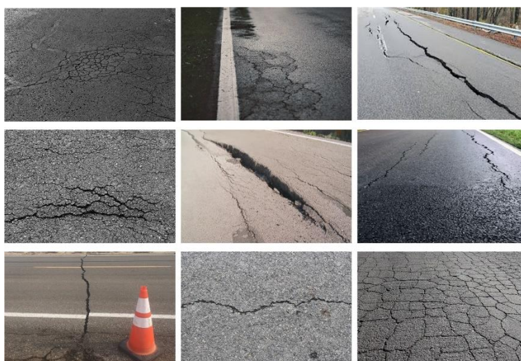
Figure 1. Examples of road crack.
