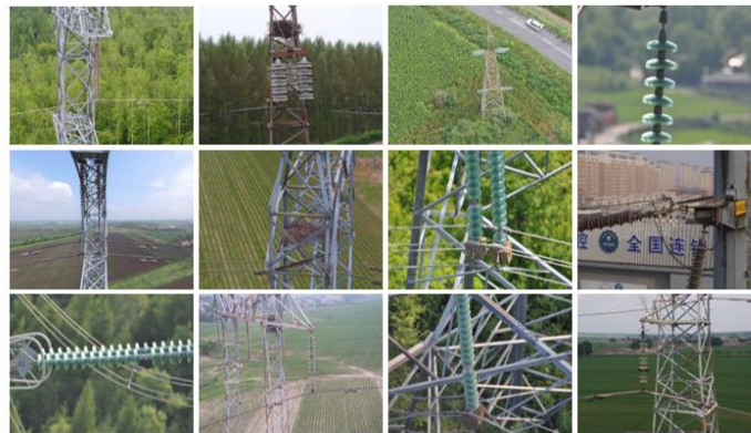
Figure 11. Insulator defect image.
