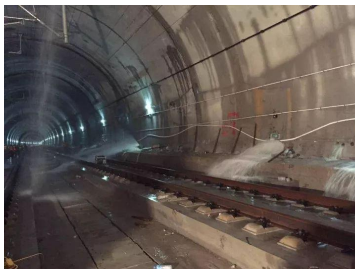
Figure 1. The example of groundwater disaster in operational high-speed railway tunnel.
